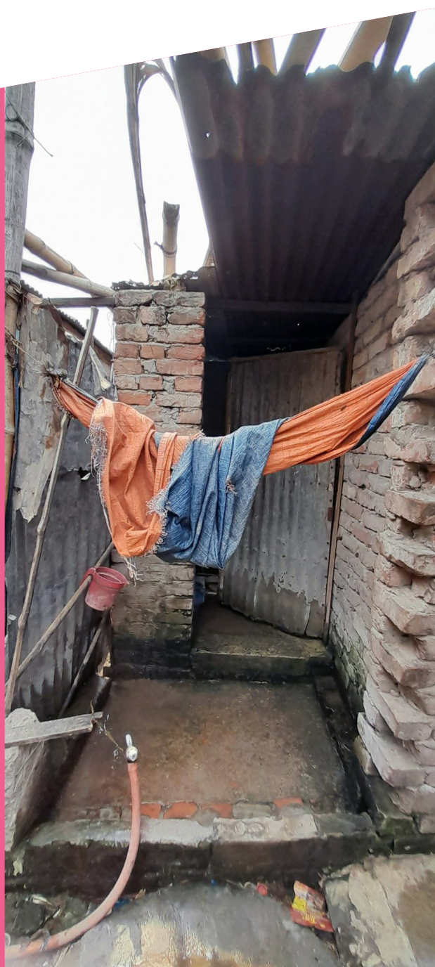
The bathroom in the building where Shapla lives is almost completely open.
